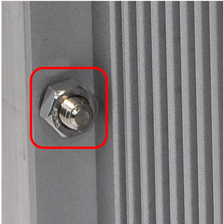
Ground screw of the switch
