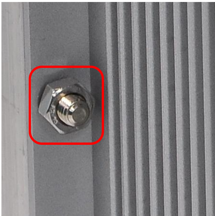
Ground screw of the switch
