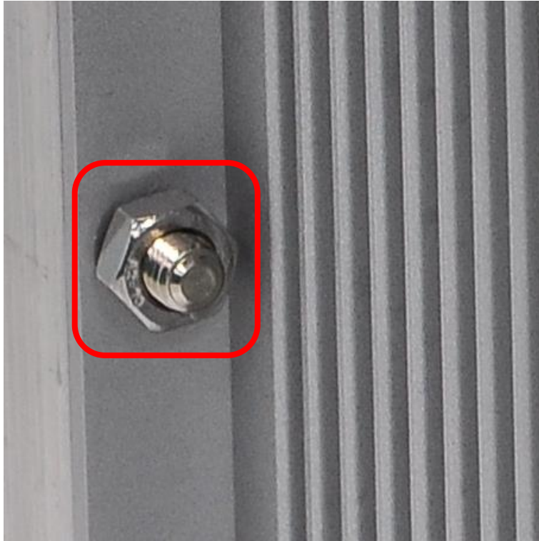
Ground screw of the switch
