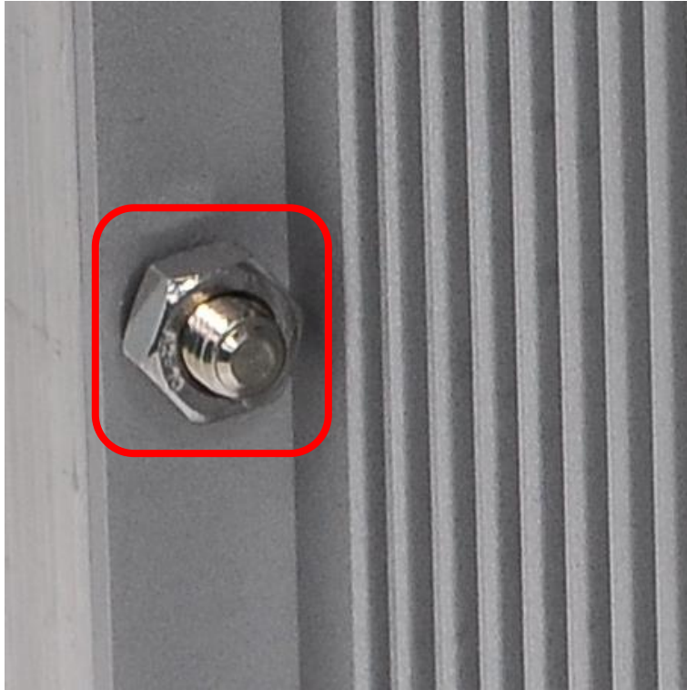
Ground screw of the switch
